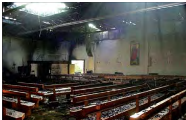
Fires from lightning strikes can cause major damage to structures
